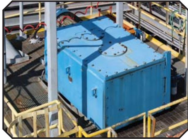
Chemineer Installed HT Agitator
