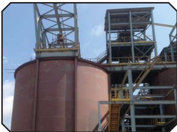
Mine Processing Infrastructure
